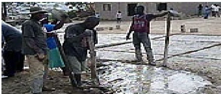
Participants clearing culverts at Yakubu Gowon Way Jos, during the Service Session
